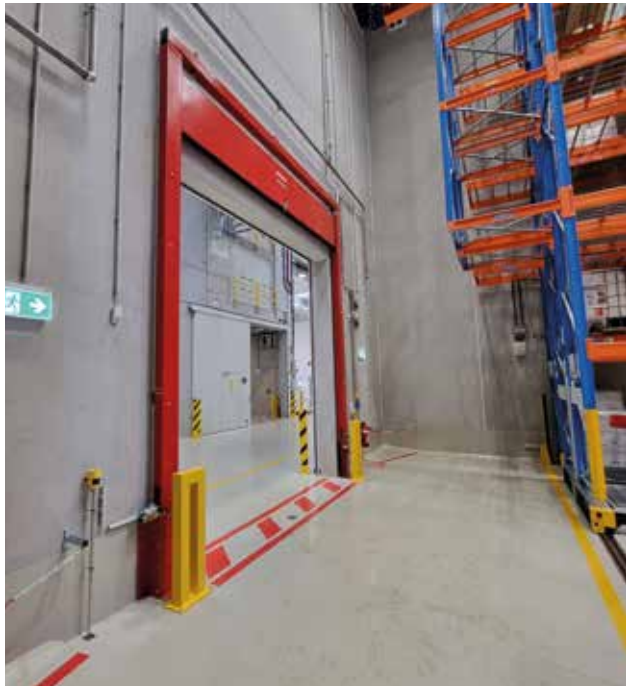
Firewater retention barriers at all exits
